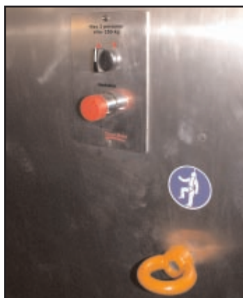
Control Panel and anchor eye attachment point for operator's safety harness when evacuating cabin in an emergency situation.
