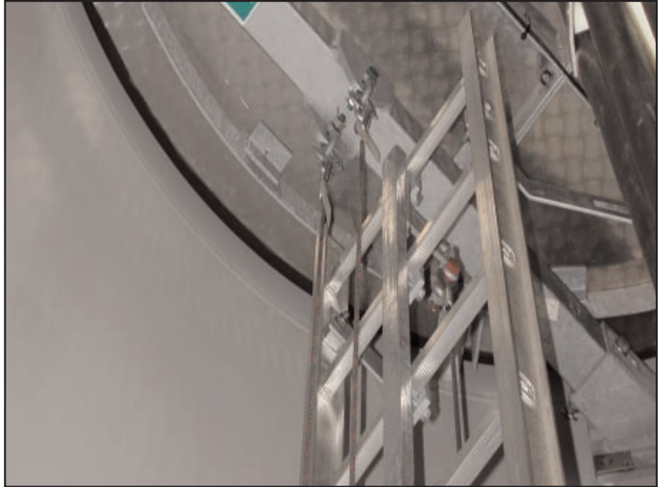
Example method of securing primary and secondary suspension cables at top of tower (interior of wind turbine). Weight at bottom keeps ropes under tension.
